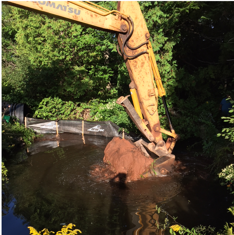
Careful excavation work on a sediment trap in the Foxley River East system.
