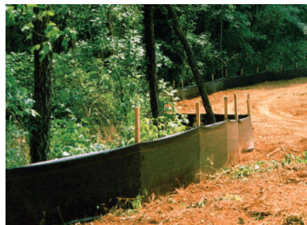
A silt fence
